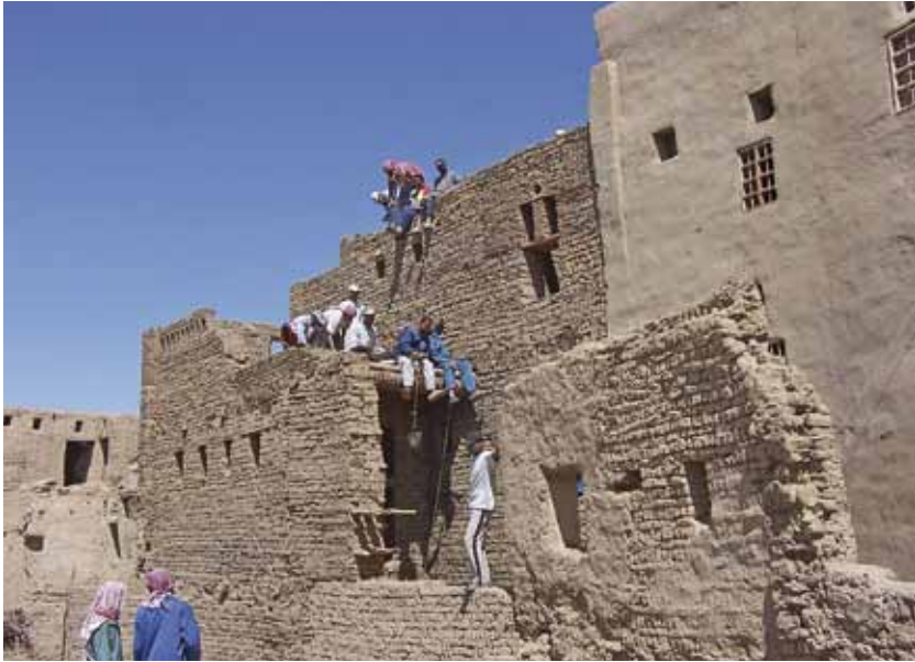
Restoration and reconstruction of traditional urban mud brick architecture in Al-Qasr in the Dakhla Oasis. Photo: Fred Leemhuis
